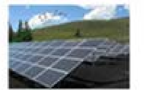
Solar power plant
