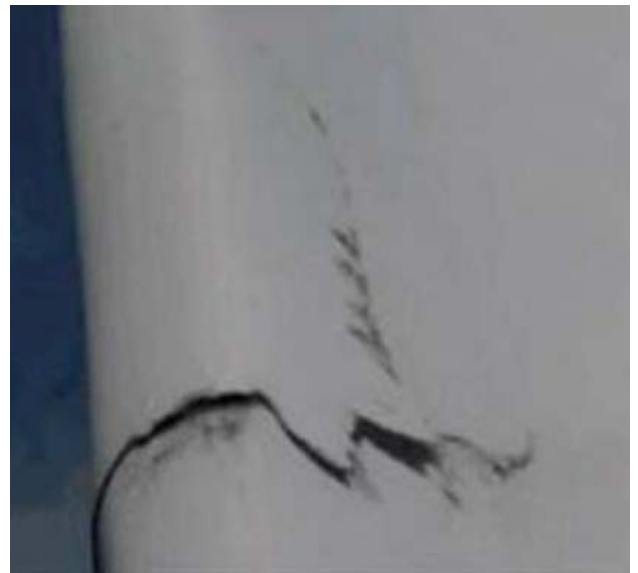
Figure B. Transverse cracks found on the trailing edge of a wind turbine blade.
